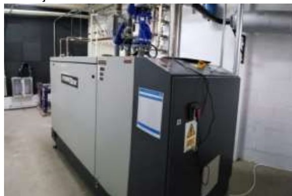
Figura 5 – CHP Powerlink 50kWe Modelo ACG50S-6NG
